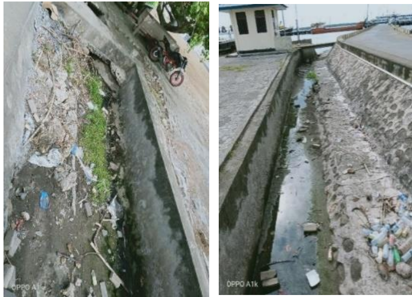
Picture 5 Faulty drainage and good drainage
